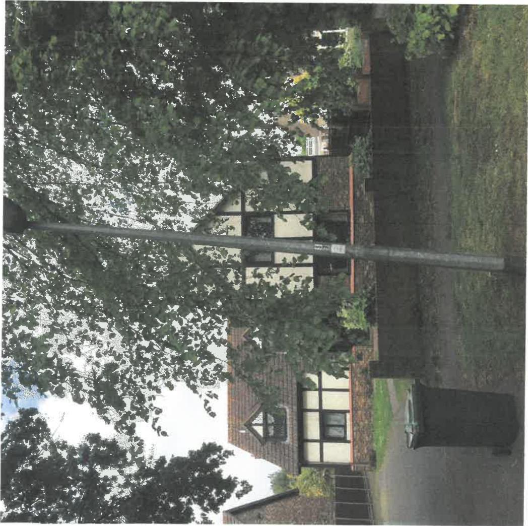
DAMAGED COLUMN S7 MILL LANE SANDY.
