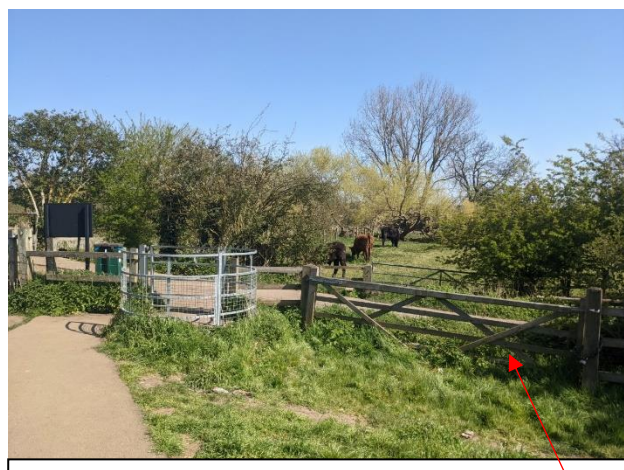
Access gate to be altered for access of long-reach machine and then repaired/replaced by IDB
